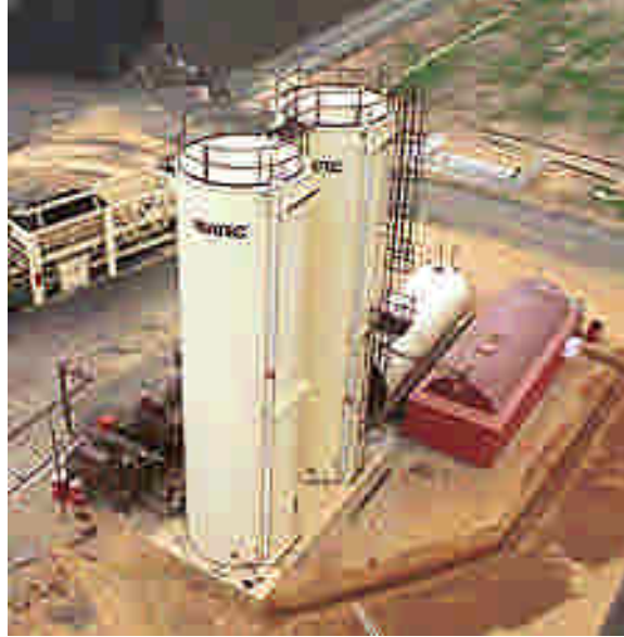
Figure 12: Vertical Asphalt Binder Storage Tanks (Courtesy Heatec, Inc.)
