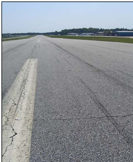
Figure 8 Transverse cracking along Runway 14-32 at Griffin-Spalding Airport
